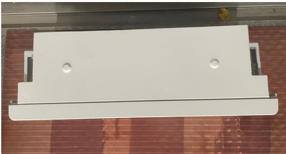
Overall view 2 of battery pack
