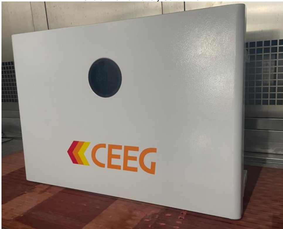
Overall view of Battery Control Box
