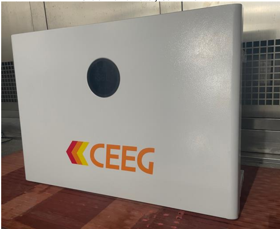
Overall view of Battery Control Box
